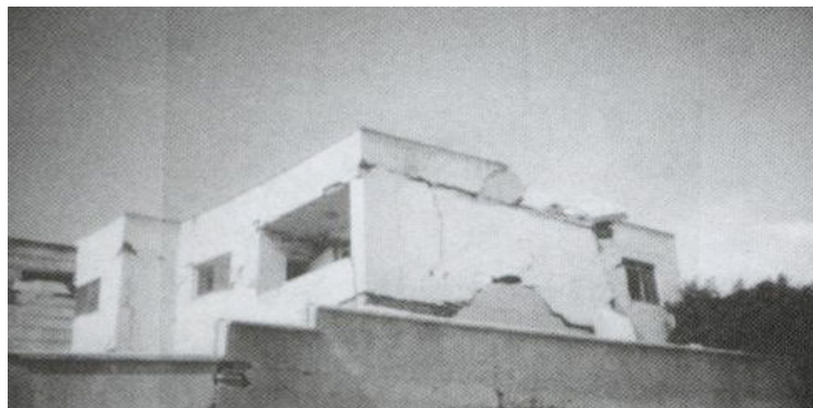
FIGURE 3. Out surface collapse of wall
