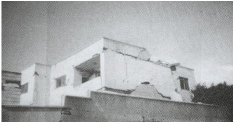
FIGURE 3. Out surface collapse of wall
