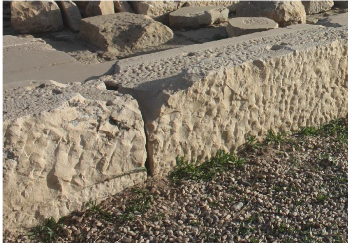
Figure 2. Example of degraded masonries in need of pointing with compatible mortars (Pasargadae, Iran)
