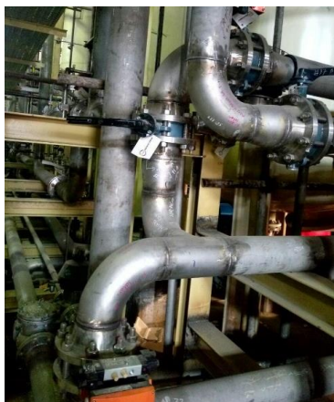
Figure 2 Piping used in Rumaila combined cycle power plant
