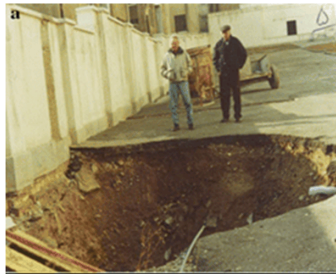
Fig. 2: Qanat collapse and its damage to structures in the north-west of Tehran (Rayhani, El Nagger, 2006).
