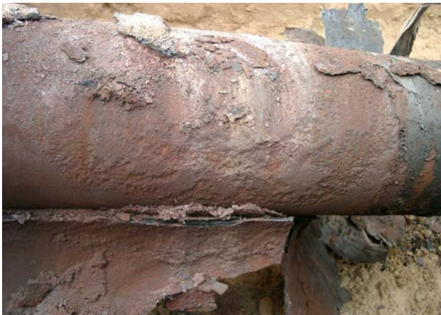
Figure 5 The HVG region of AL99A pipeline and the shape of corrosion
