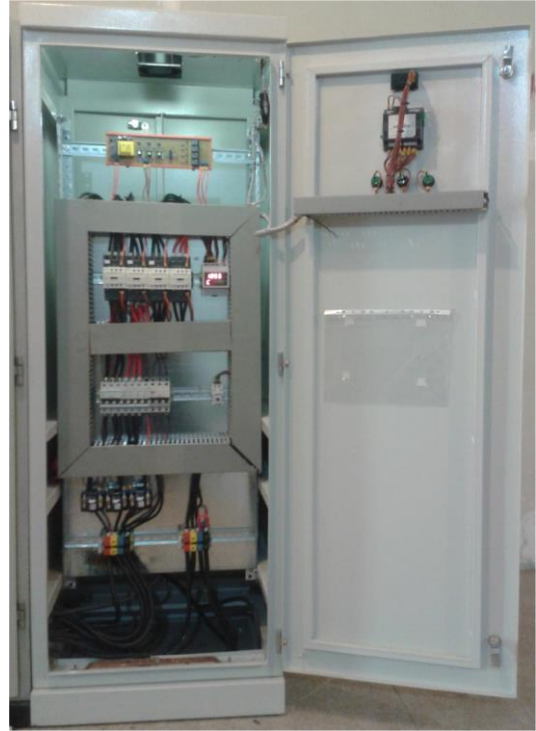
Fig. 6. Frontal view of the intelligent lighting control panel
